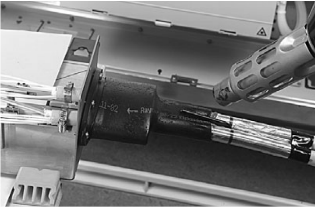
5.4.12 Heat until the green thermo-indicating paint has changed to black and the hot melt adhesive (yellow) in the clip area is mixed with the sleeve adhesive (red).
