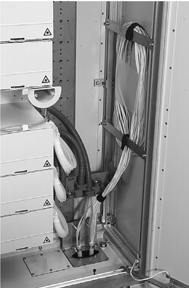
5.4.13 Mount the cable and plate in the cabinet. Secure the loop behind the metal bars using the Velcro strips.
