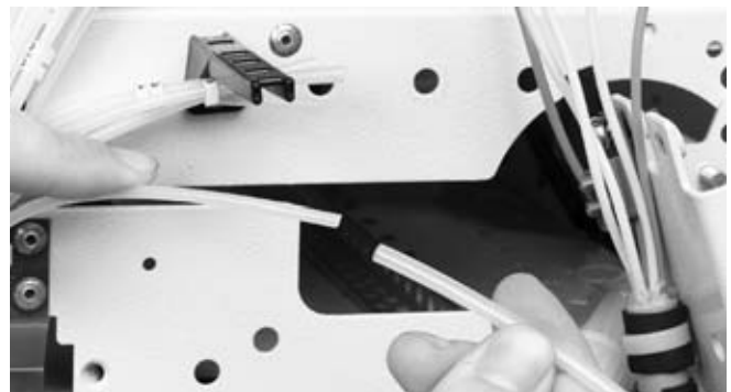
4.2.7 After stripping the loose tubes and cutting of the overlength of the transportation tubes, slide the FOPT-CT over the transportation tubes. Clean the fibers very well to make feeding easier.
